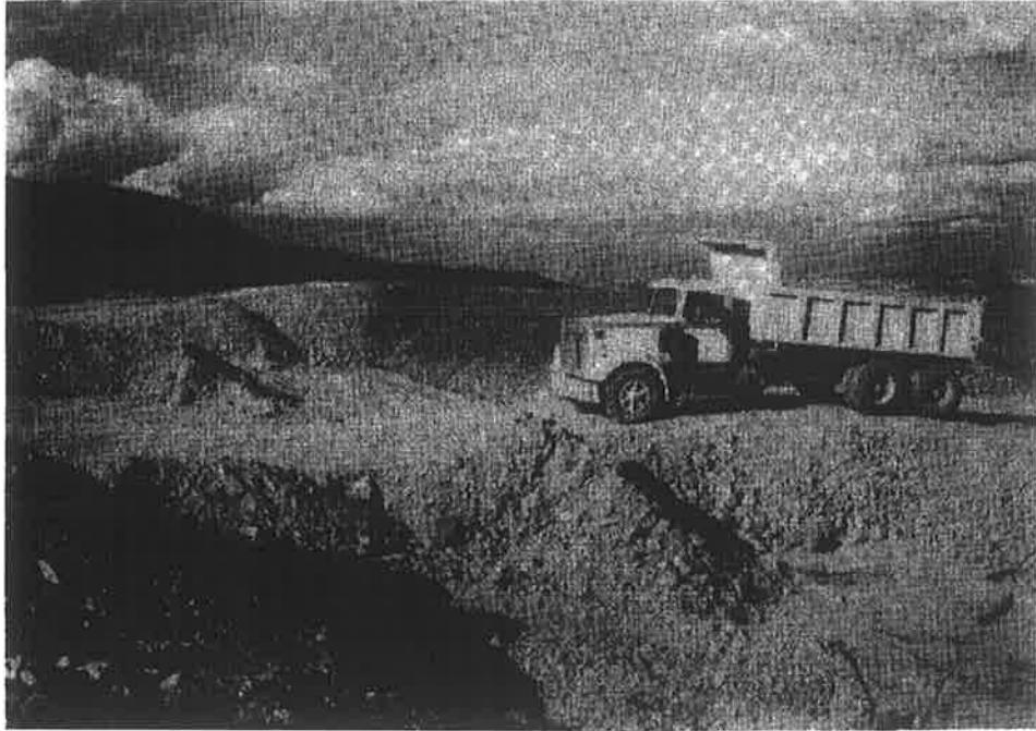
Figure 10. Heaps are built in three 5-foot lifts. The heap in the background will remain under leach for at least two months. The first layer of the adjacent heap is under construction in the foreground.
