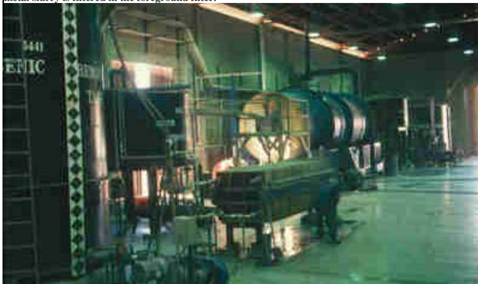
Figure 4. Precipitation drum and precipitate filter. Two tonnes per day of scrap iron are added to the discharge end of the drum. Drum discharge is pumped to a thickener behind the plant and the thickened metal slurry is filtered in the foreground filter.
