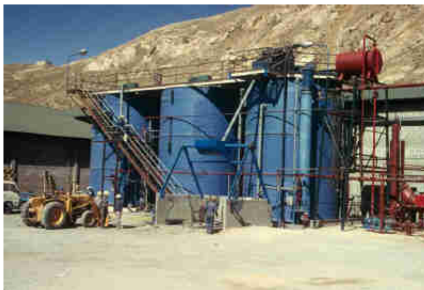
Figure 3 Ore Slurry is fed to the leach tanks at 45% solids. Leach tanks are rubber lined and externally insulated. The system that is barely visible on the right hand side of the photo is a hot thermal fluid heater used to raise the process solution to 75°C.
