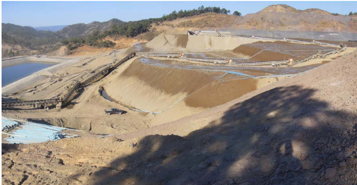
FIGURE 6. THE STACKING SYSTEM IS NOW ON AN UPPER LEVEL. IT ADVANCED WHILE STACKING UP A SPIRAL RAMP, AND IS SHOWN ADVANCING ON A LEVEL SURFACE, 10 METERS ABOVE AN EARLIER BENCH. LEACH PIPES ARE REMOVED AS THE HEAP ADVANCES OVER THE OLDER MATERIAL.
