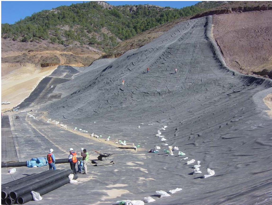
FIGURE 4. SIDESLOPE LINER CONSISTS OF A GEOTEXTILE LAYER, A LAYER OF GCL (CLAY ENCLOSED IN GEOTEXTILE), AND A TOP 60 MIL HDPE COVER.
